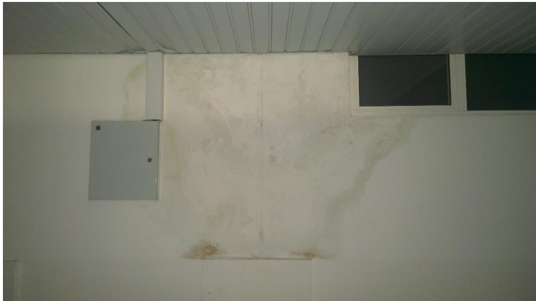
Figure 4.1: Dampness on the Upper Section of the Wall Due to Rain Penetration. Civil Engineering Department, Eastern Mediterranean University (EMU), Mağusa, North Cyprus.
