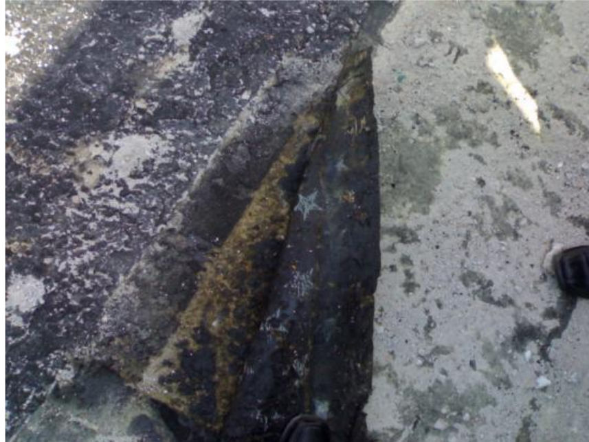
Figure 4.5. Failed Torch-on Membrane at Social Security Organisation (SOC SO) in Seberang Jaya, Malaysia (Suffian, 2013).
