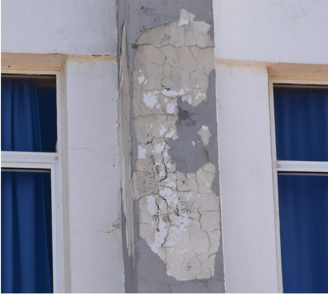
Figure 4.3: Map cracking on the Column of the Top Floor That Led to the fall of some of the Paint Cover. English Preparatory School, Eastern Mediterranean University, Mağusa, North Cyprus.
