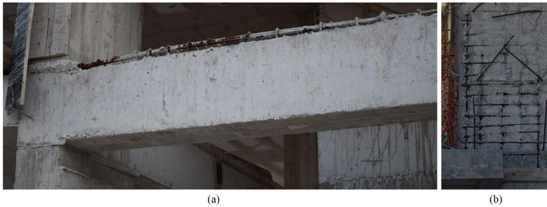
Figure 3.9: Shifted Reinforcing Bar Cages in: a Beam (a) and in a Sheer Wall (b). Residential Buildings, Mağusa, North Cyprus. (Case Study #111 (Page 203)).
