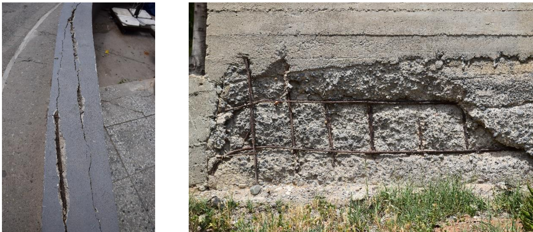
Figure 3.5: Cracks and spalls in concrete short walls. Public structures, Mağusa, North Cyprus.
