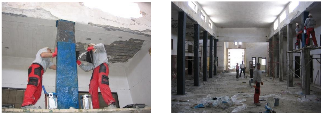
Figure 3.7: Strengthening of the Old Bazaar by Using CFRP in İskele, North Cyprus (Naimi and Celikag, 2010)
