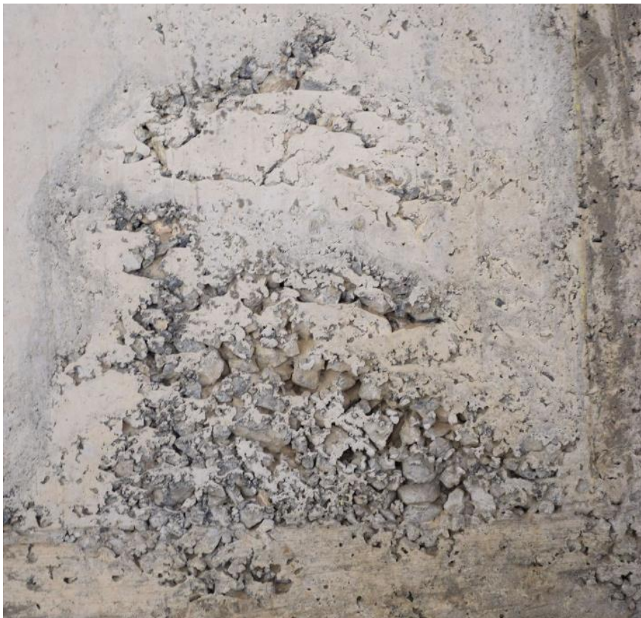
Figure 3.16: Honeycomb in a Column. Residential Building, Magusa, North Cyprus. (Case Study #104 (Page 196)).
