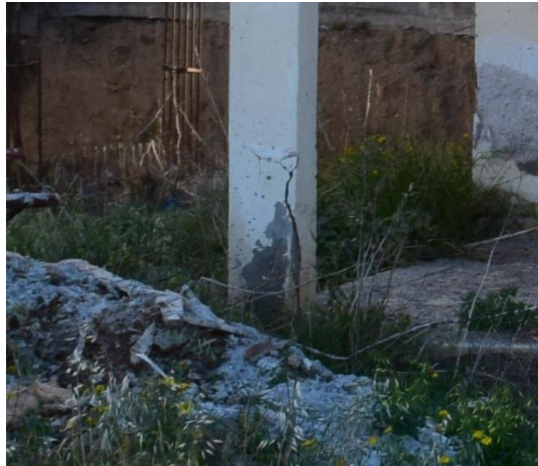
Figure 3.2: Corrosion Crack in the Lower Part of a Column. Mağusa, North Cyprus. (Case Study #1 (Page 93)).
