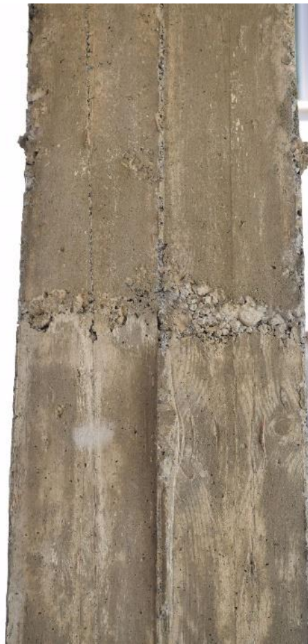
Figure 3.13: Cold Joint in Column. Residential Buildings, Mağusa, North Cyprus. (Case Study #104 (Page 196)).
