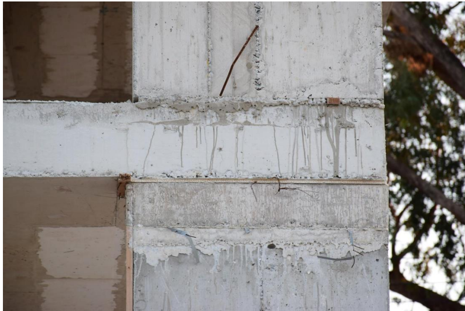
Figure 3.14: Cold Joint Between Column and Slab. Residential Buildings, Mağusa, North Cyprus. (Case Study #111 (Page 203)).
