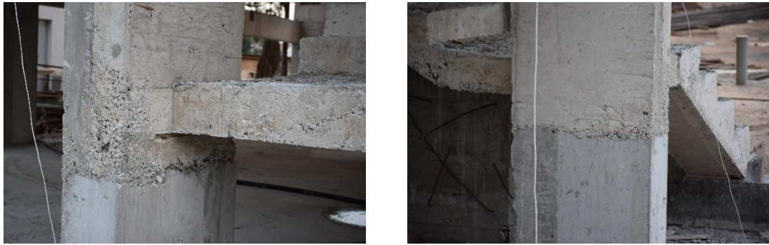
Figure 3.12: Cold Joints in Columns. Residential Buildings, Mağusa, North Cyprus. (Case Study #111 (Page 203)).
