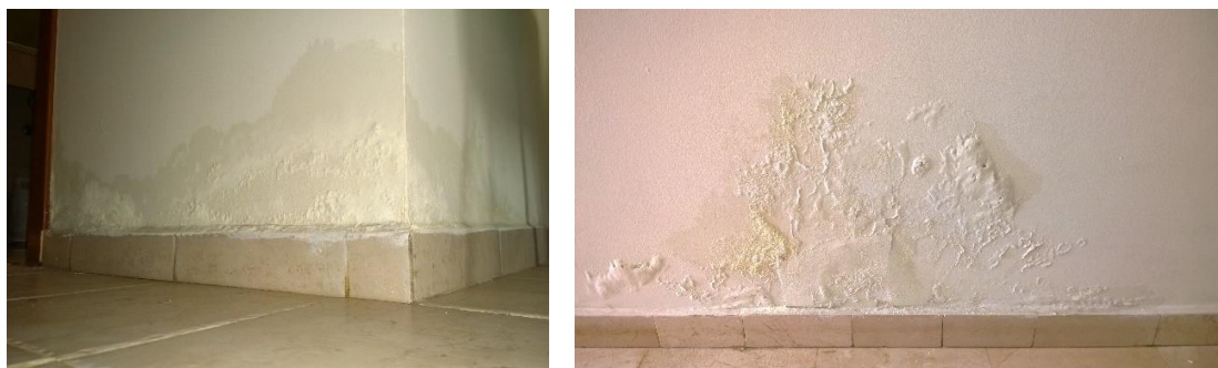
Figure 4.2: Dampness on The Lower Part of Second Floor Walls Due to Wet Floors Caused by Frequent Floor Washing Using Too Much Water Which Can Be Mistaken Easily as Rising Damp. Akdeniz Gormitory, Eastern Mediterranean University (EMU), Mağusa, North Cyprus.
