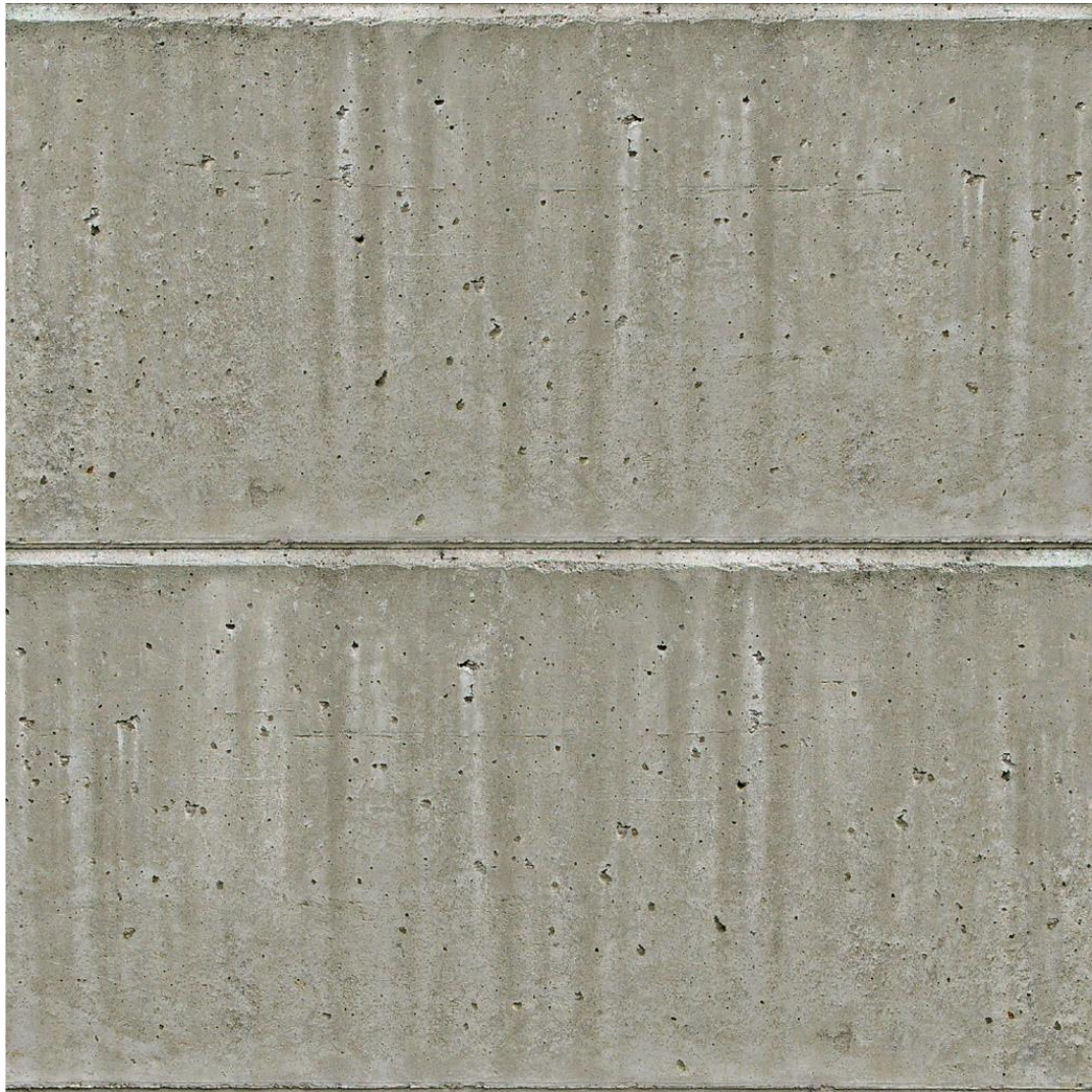
Figure 4.4: Efflorescence on Concrete Surface.
