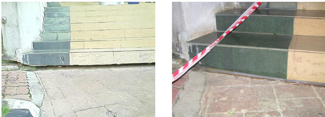
Figure 2.23: Before (on the left) and After (on the right) the Treatment Using Resin Injection at Social Security Organisation (SOCSO) Building in Penang, Malaysia (Suffian, 2013).
