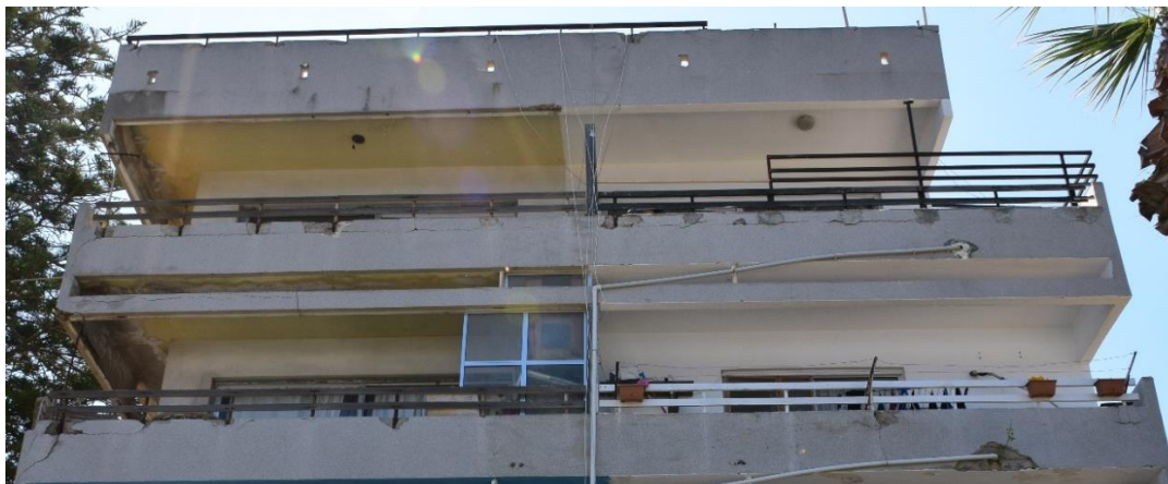
Figure 3.4: Cracks Due to Dissimilar Metal Corrosion around Handrail's Embedded Metal Balusters of Balconies. Residential Building, Palm Beach, Mağusa, North Cyprus. (Case Study #24 (Page 116)).
