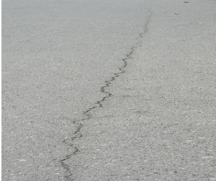
Figure A2. Longitudinal & Transverse Crack
