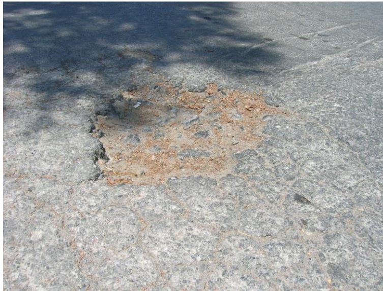
Figure A4. Pothole
