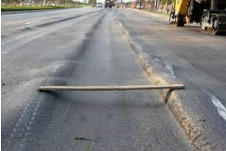
Figure A5. Rutting, (BMT, 2013)
