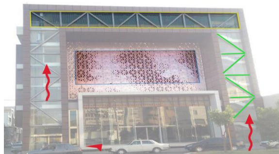
Figure 109: Façade analysis, its form-active structure has efficient side and top trusses which are technically and visually working
