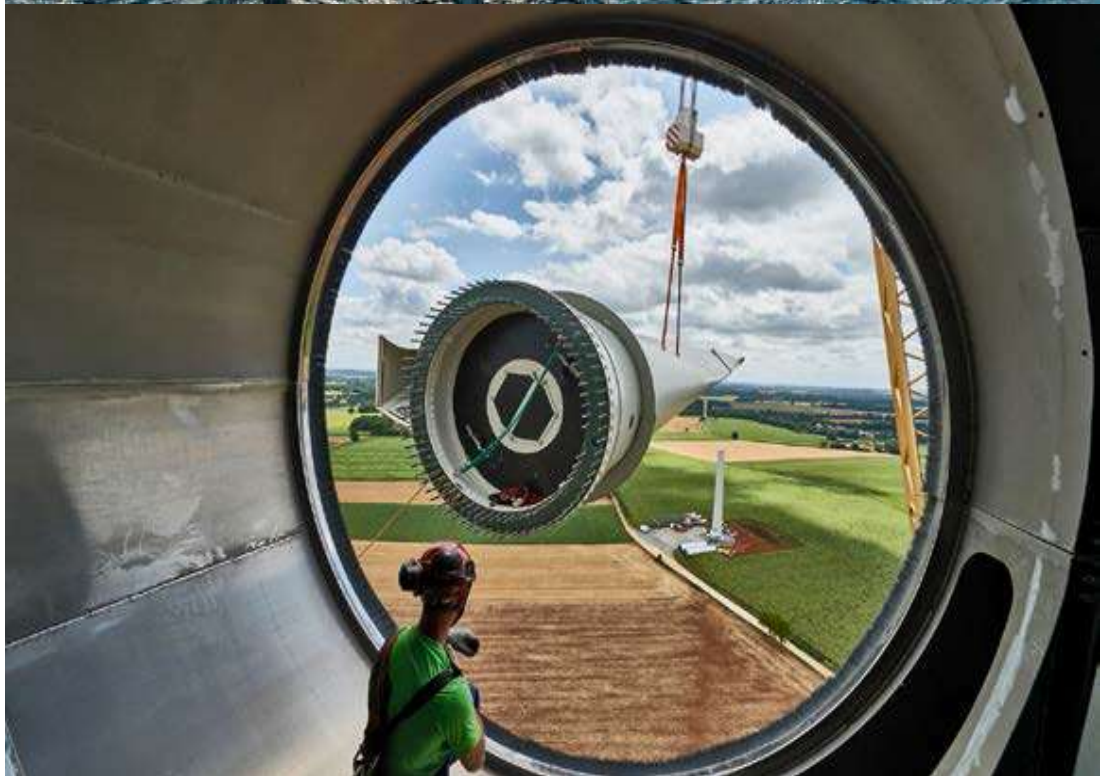
Figure 2.8: Part of assembling procedure for off- and on-shore wind farms in Europe
