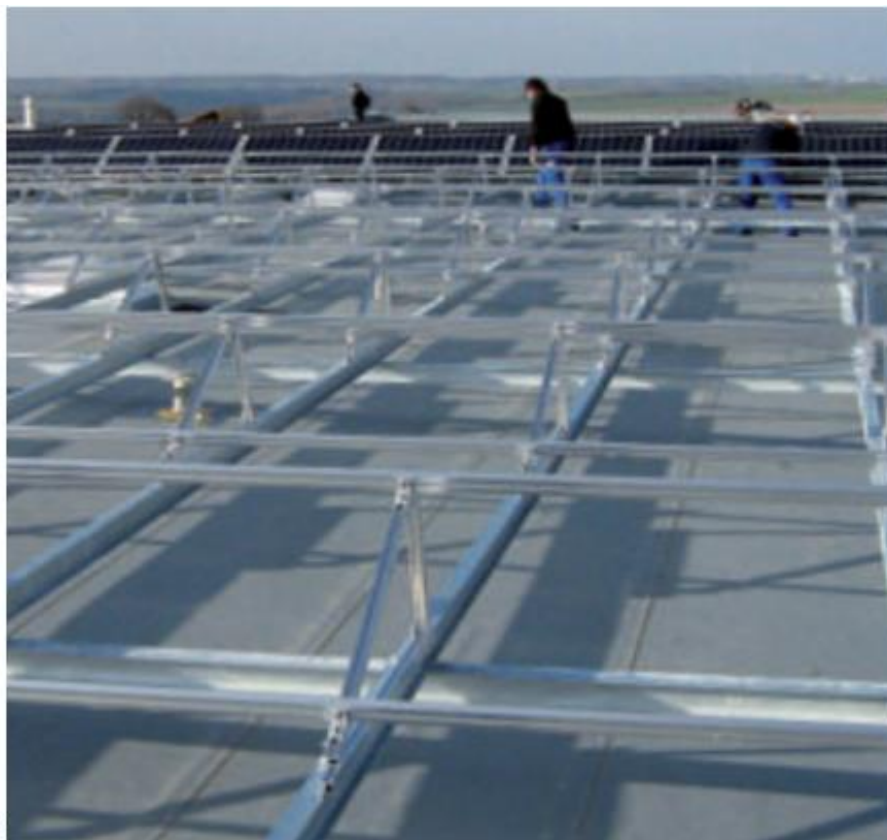
Figure 3.6. PV on roof with tubular section ( http://www.greenbuildingenergysavings.com )
