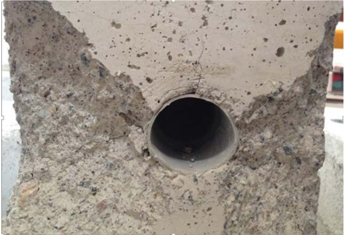
Figure 3.16. Spalling of concrete at exit location
