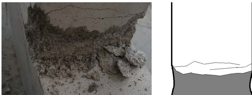
Figure 5.8. State of column C-9 after the test
