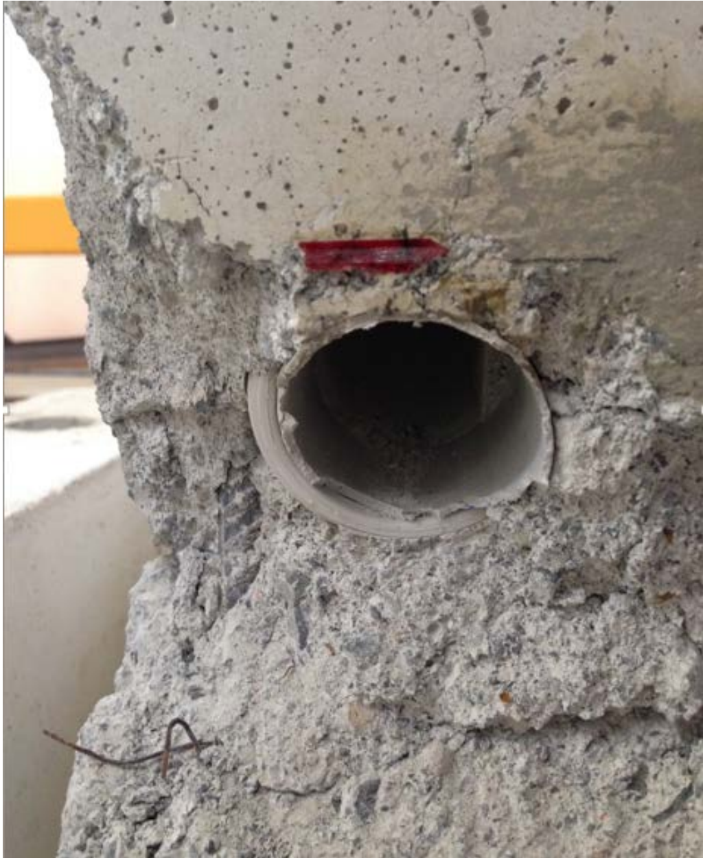
Figure 3.15. Severe damage at exit location in specimen C-4
