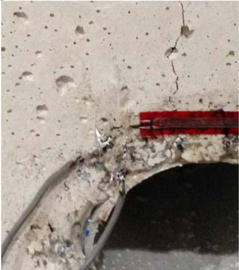
Figure 3.17. Tension crack above the exit location observed in early stages of loading
