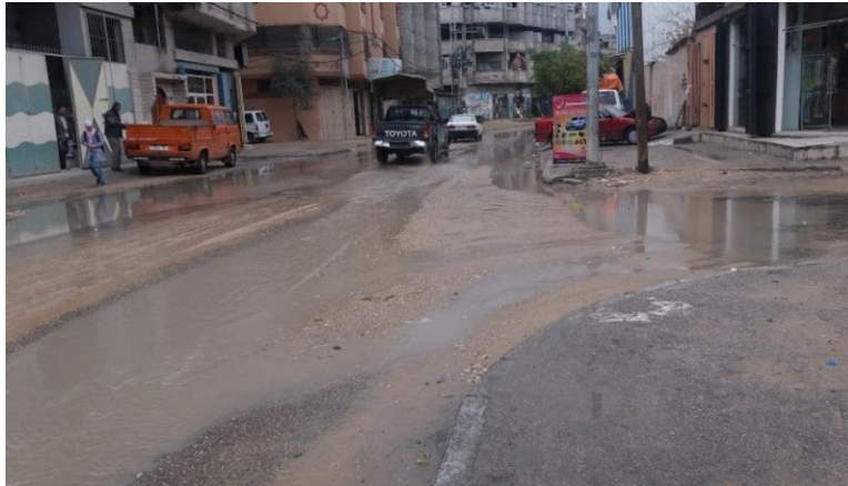
Figure 33: Poor Condition Road in the City of Gaza Photo Retrieved from (URL20)
