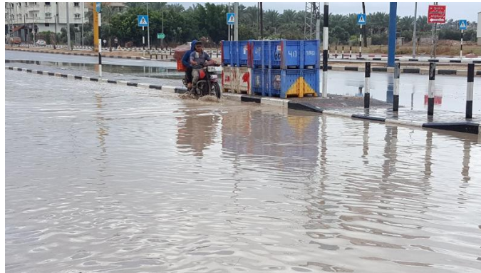
Figure 35: Damaged Street Infrastructure in Gaza City Retrieved From (URL22)
