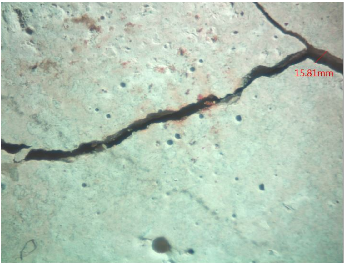
Figure 44e: NSC-40% PP surfaces after 200 °C heating at 28 days
