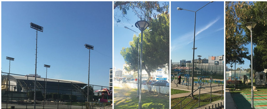
Figure 25. Existing lighting elements.
