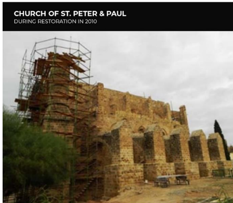
Figure 4.27: Church of St. Peter and Paul during the restoration process in 2010 (Yüceer, 2012)
