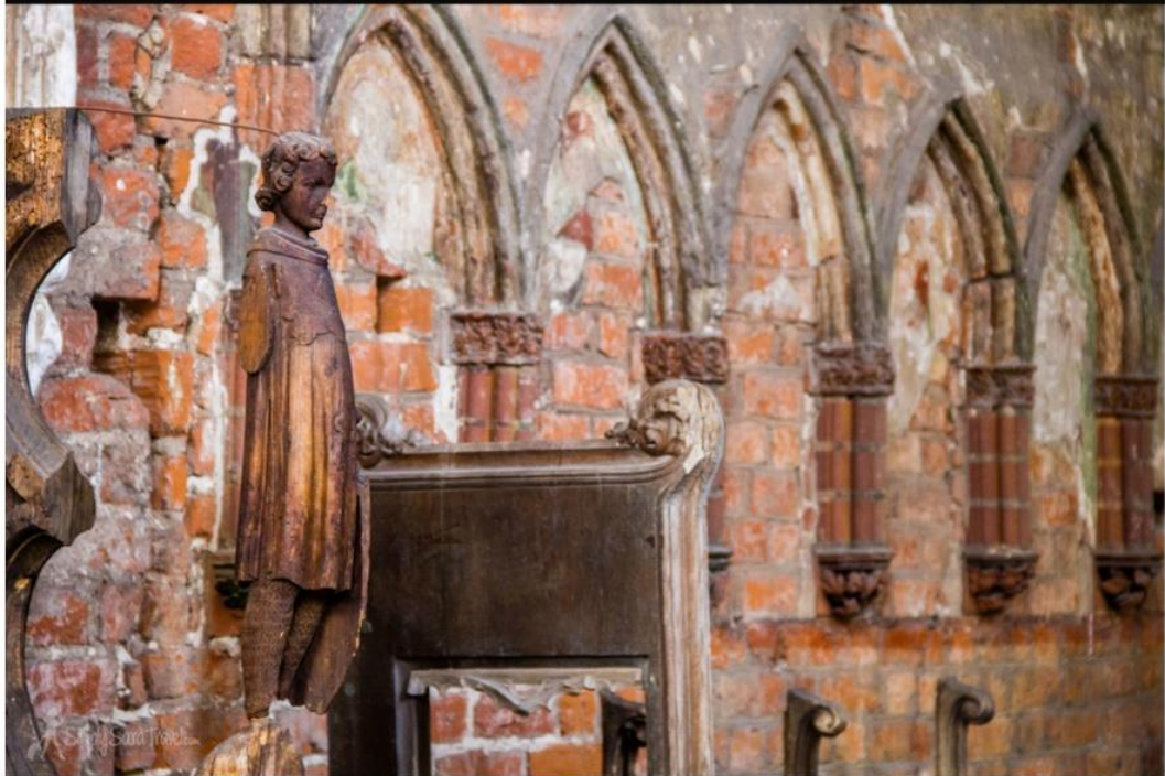
Figure 4.17: A detail showing the preserved damaged walls (Malbork Museum, 2021)
