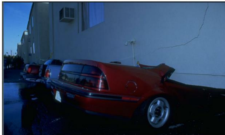
Figure 7: Collapse by soft story in the Northridge earthquake 1994 [20]
