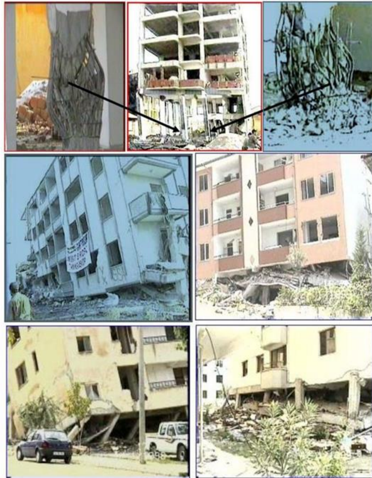
Figure 8: Soft story destruction Izmit earthquake in Turkey 1999[18]
