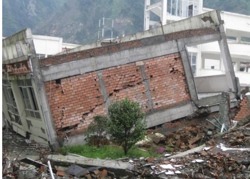
Figure 9: Soft story collapse 2008 Wenchuan earthquake in China[22]
