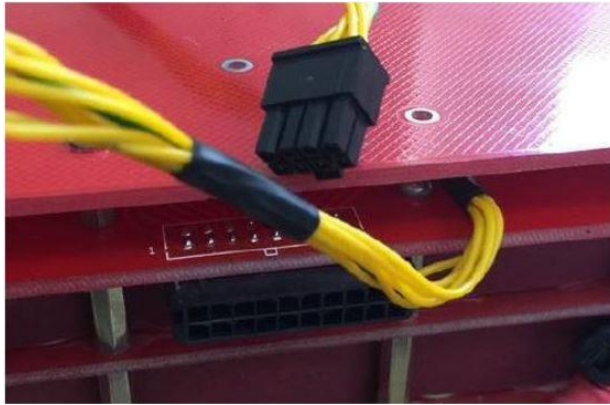
Figure 17: Temperature and BMS Circuitry Connector Outlet
