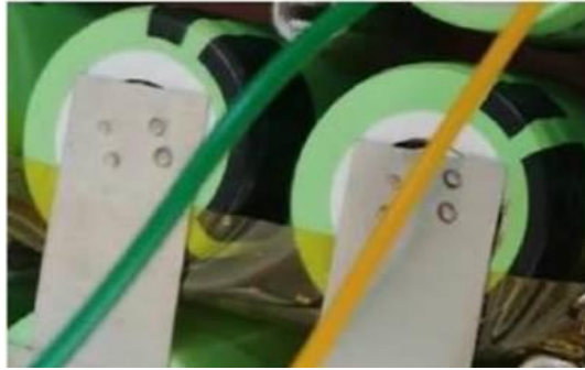
Figure 15: Cell Connection inside Battery Pack
