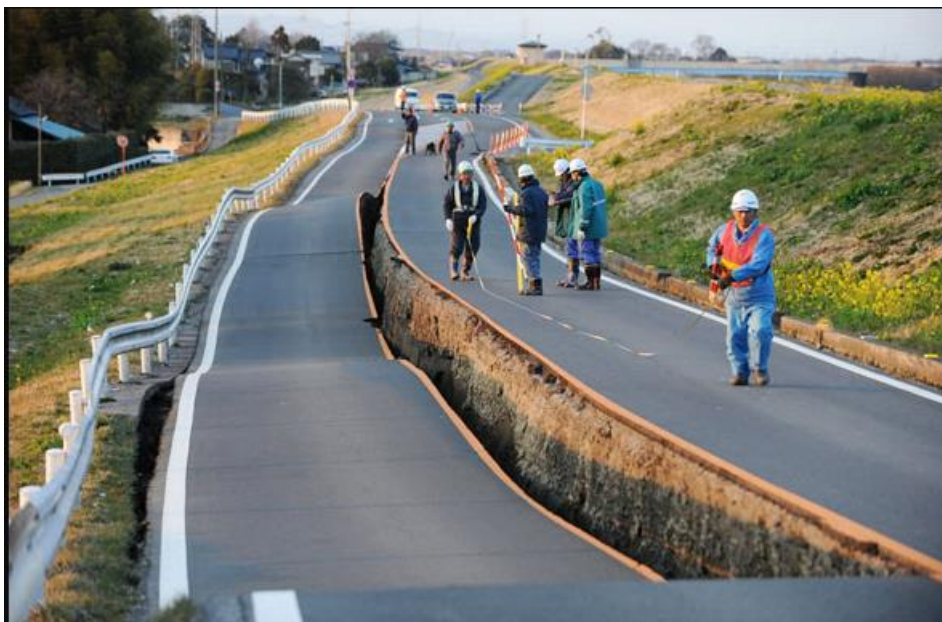
Figure 3: Lateral spreading Joban Motorway Japan 2011, M_w = 9.0 (Dillerstone, 2011).
