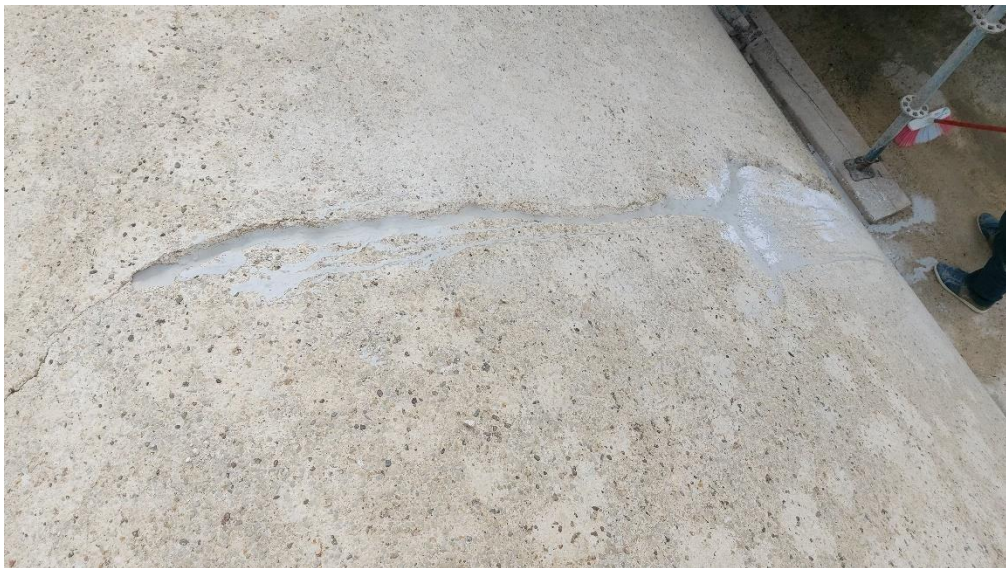
Figure 2.9: Cracks at roof
