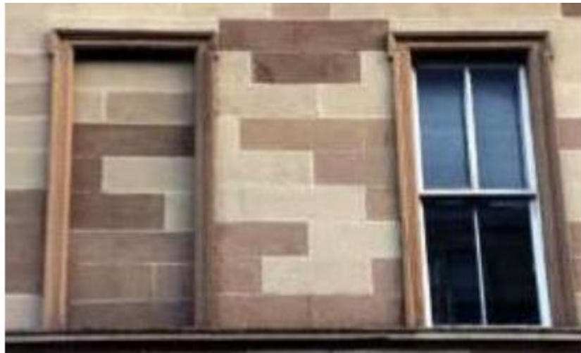
Figure 2.66: Example of mortar application (light parts) as a mortar repair of deteriorated stone units in Glasgow. Scotland [24]
