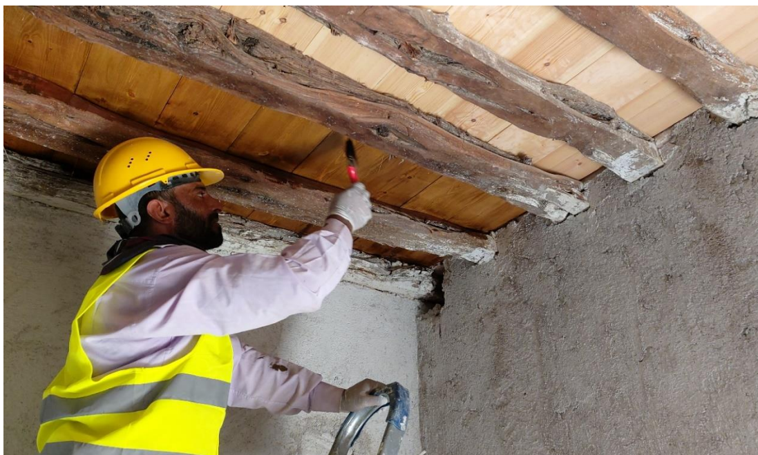
Figure 2.51: Cleaning of beams and parapet with paint-remover and applying of water-based varnish
