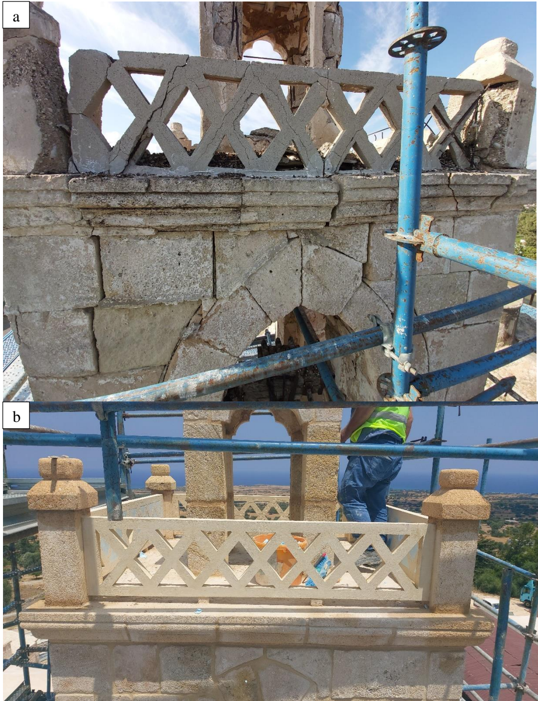
Figure 2.37: a) Initial condition b) Construction of new stone rail and corner posts
