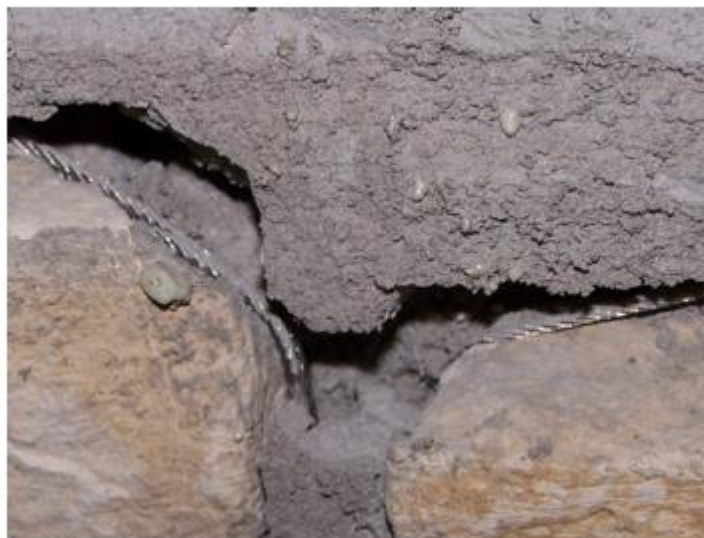
Figure 2.71: Stainless steel cord inside opened three leaf masonry wall joint [25]
