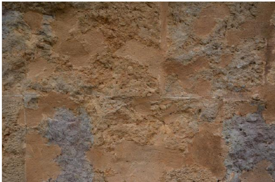
Figure 2.69: Mortar repair carried out on multi-coloured degraded sandstone blocks Palazzo Piccolomini, Pienza, Italy [24]
