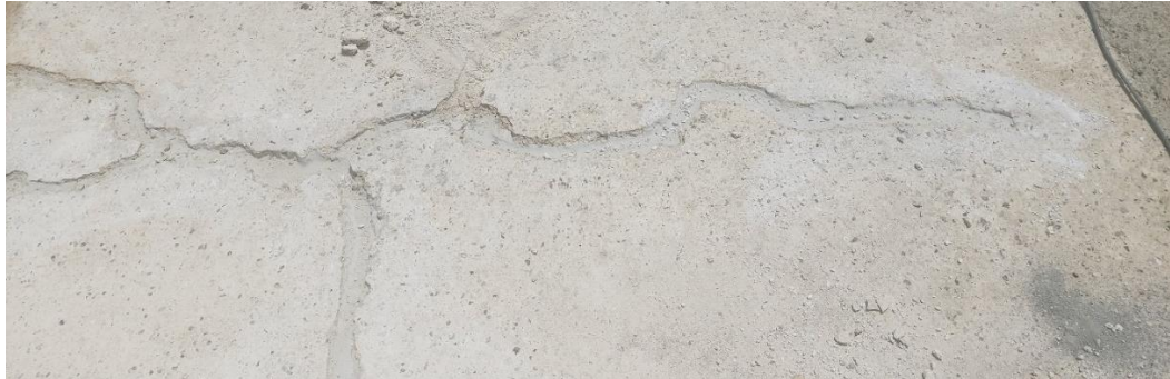
Figure 2.8: Cracks at roof
