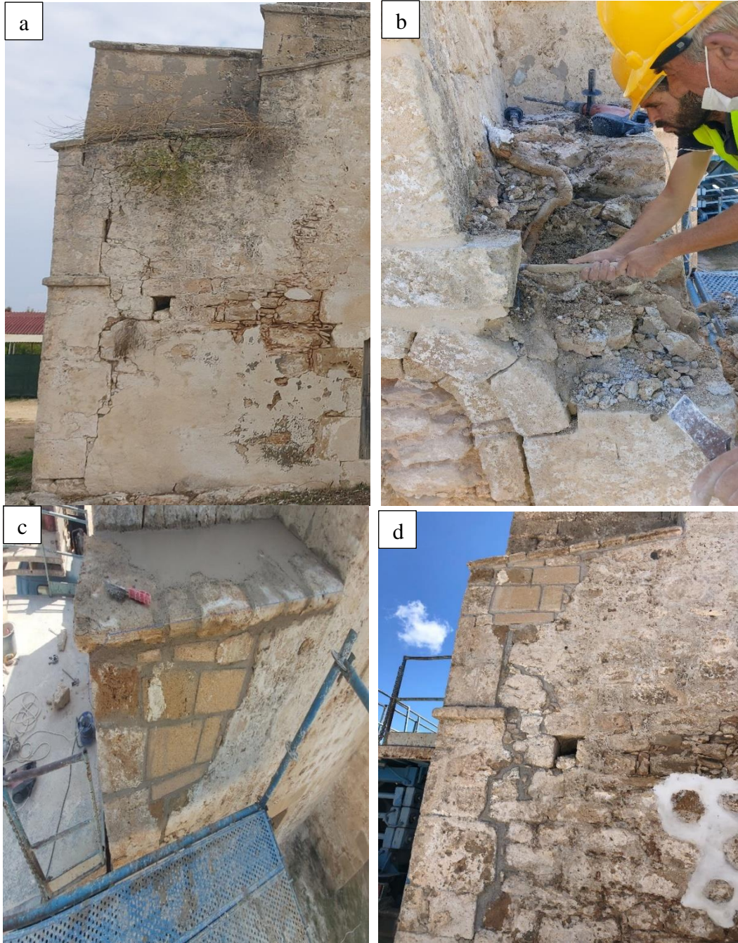
Figure 2.33: a) Dismantling and rebuilding of seriously damaged part stage 1 b) Stage 2 c) Stage 3 d) Stage 4
