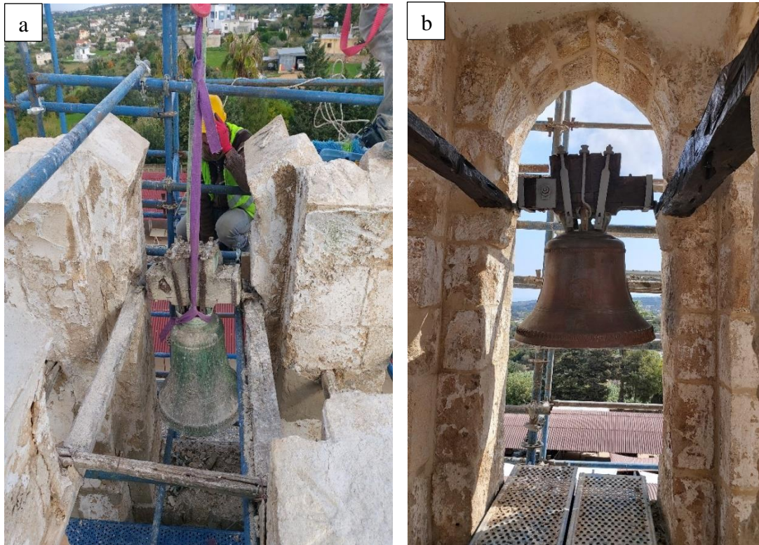
Figure 2.43: a) Initial condition of bell b) Bell and its' mechanism were removed and repaired
