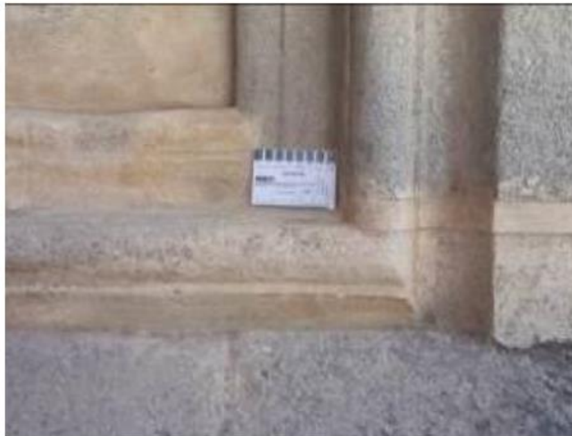
Figure 2.67: Mortar used to repair deteriorated stone parts and detailing of the main entrance portal of the cathedral in Évora. Portugal [24]
