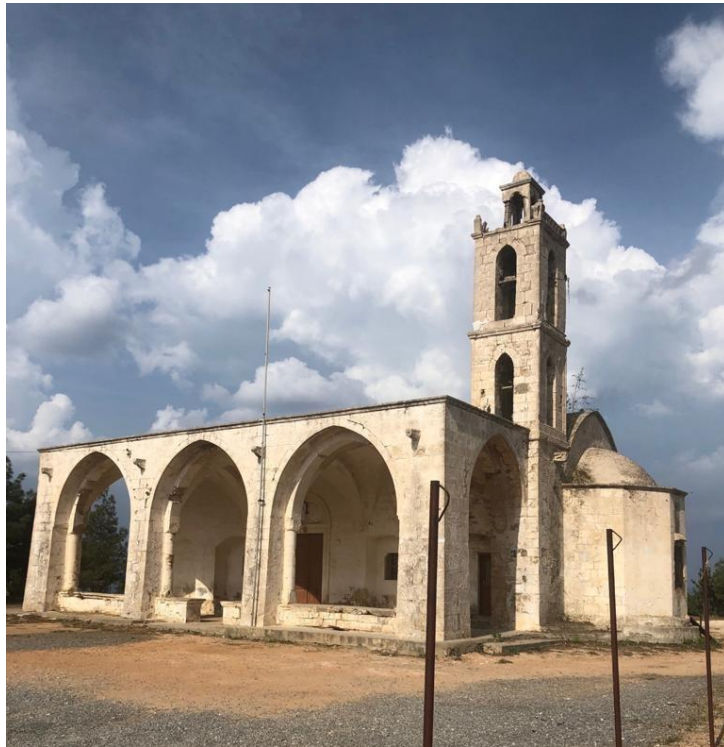
Figure 2.2: Archangelos Michael Church, view of the southern side (new part) before conservation works
