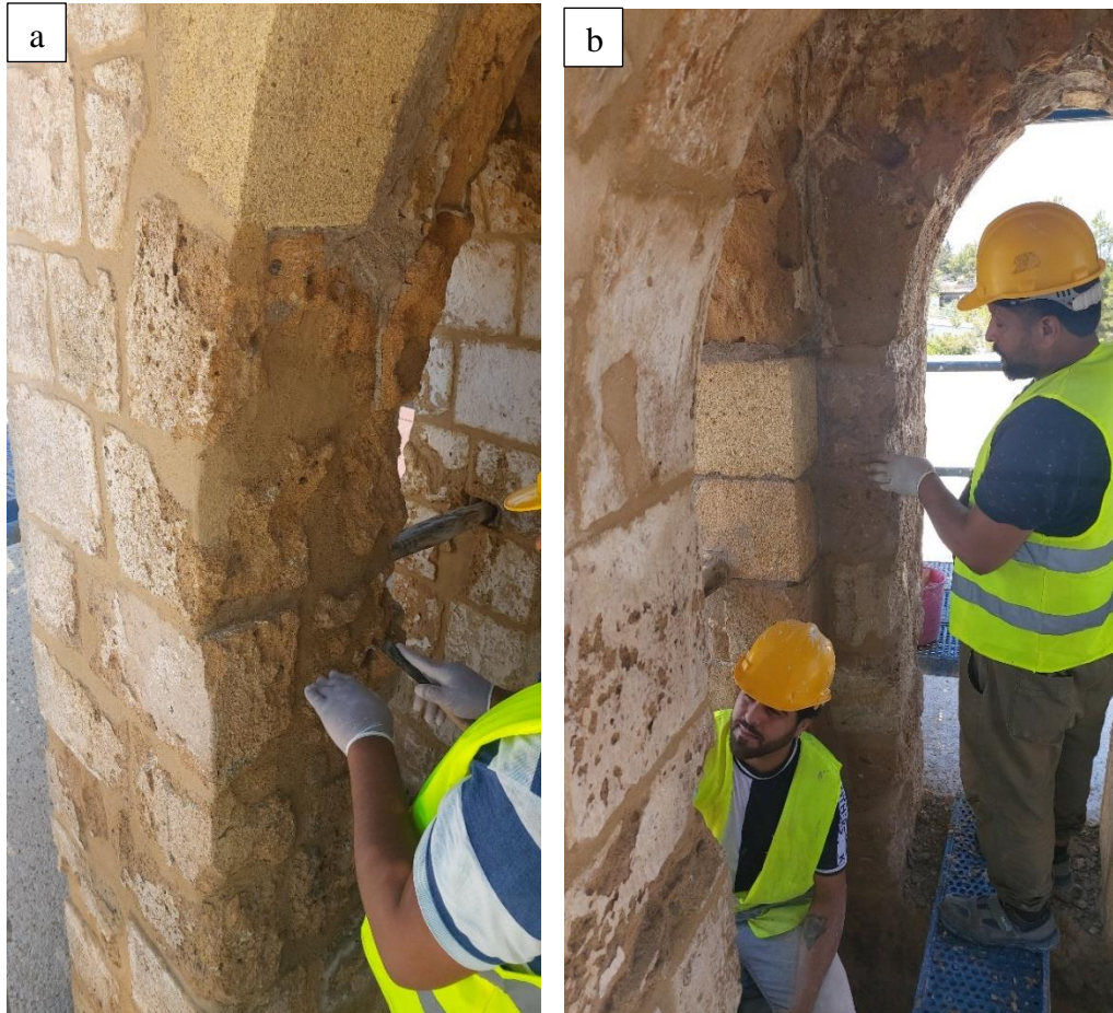
Figure 2.41: a) Repairing internal sides of columns 1 b) Replacing of internal sides of columns 2
