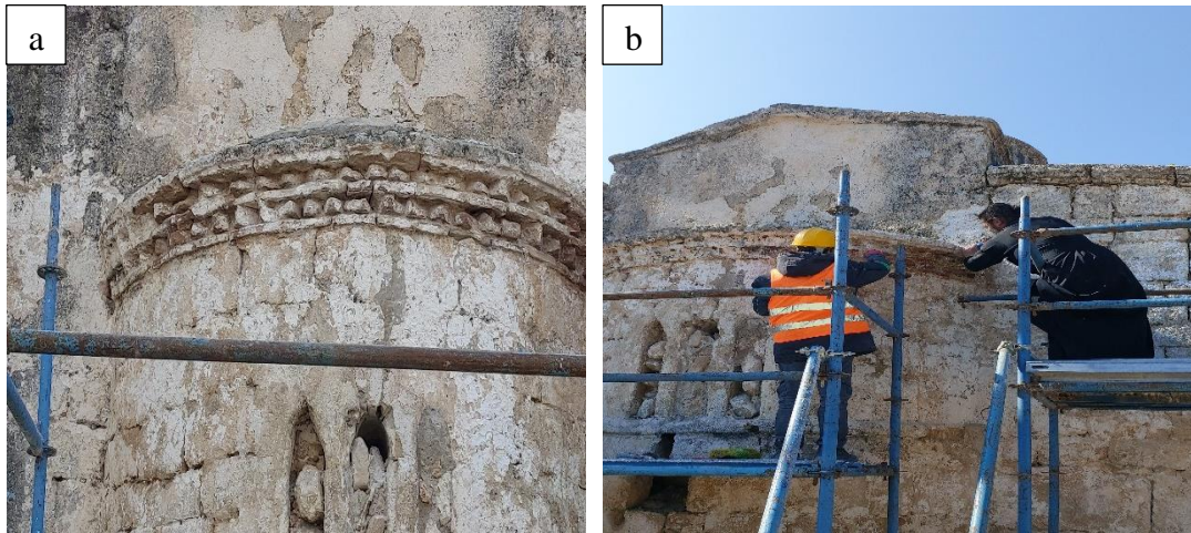
Figure 2.3: a) Initial condition b) Removal of plaster from external walls of the church
