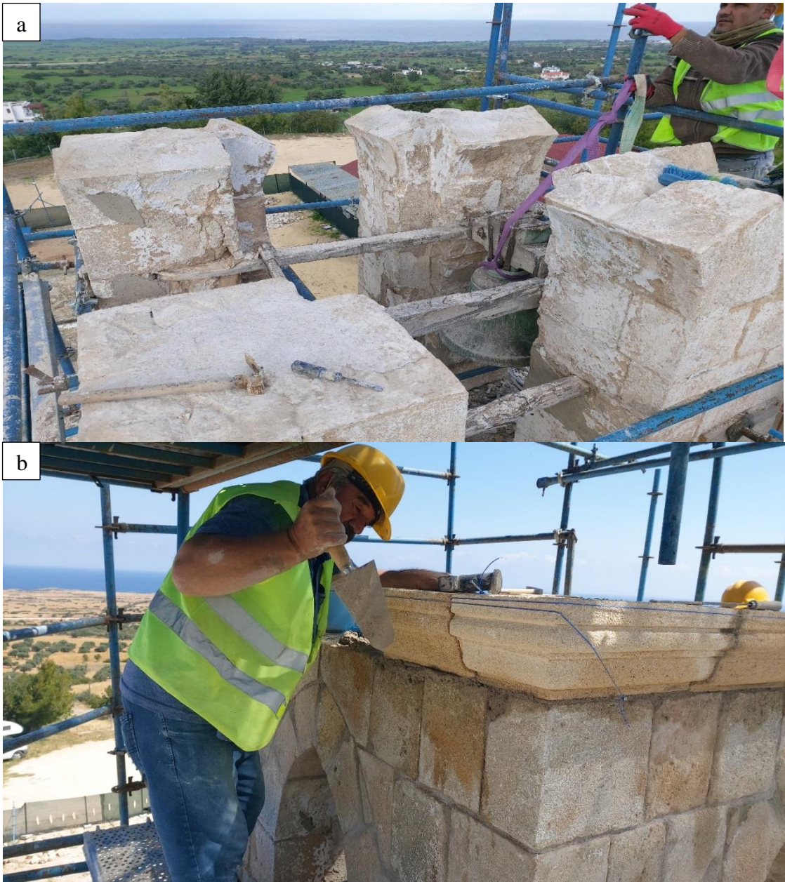
Figure 2.36: a) Dismantled condition b) Adding new cornice stones at 23 th row of belfry
