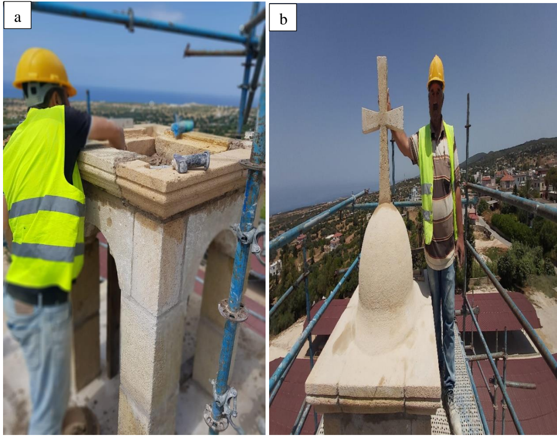
Figure 2.38: a) Rebuilding of new stone columns and arches b) Rebuilding of new stone coupole
