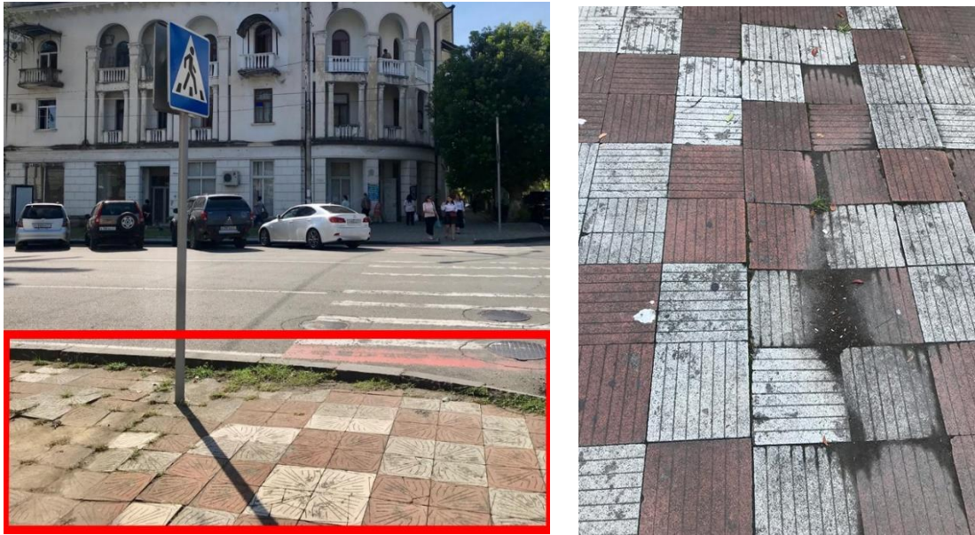
Figure 35: Pictures show the absence of ramp and special materials for disabled people.
