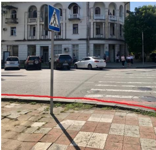
Figure 54: Poor condition of sidewalk.
