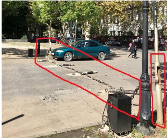
Figure 49: Bumps and light poles in poor conditions.
