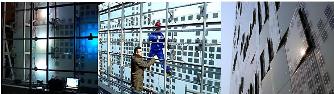
Figure 33: The cladding structure detail of Media Wall (Robert and Guariento, 2009) and ( http://www.greenpix.org/download.php ).
