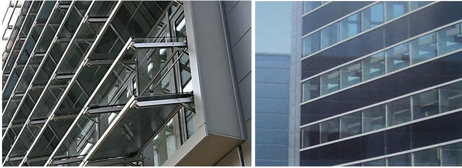
Figure 66: Opened and closed view of PV modules of Würth Solar CIS Factory's façade in Schwabisch Hall, Germany (Lüling, 2009).
