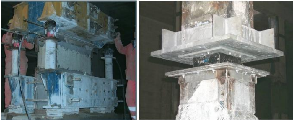
Figure 9: Column before and after the installation of the isolator (Clemente et al. 2012)
