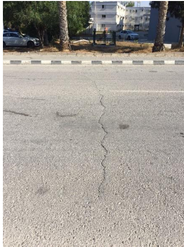
Figure 11: Moderate severity transverse crack
