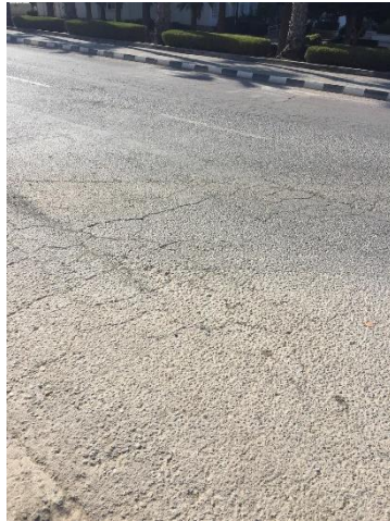
Figure 3: Moderate severity alligator crack
