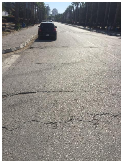
Figure 12: High severity transverse crack
