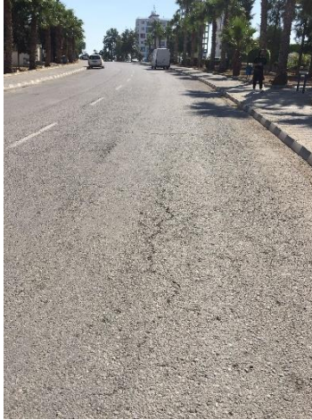
Figure 2: Low severity alligator crack
