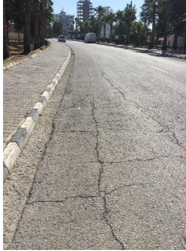
Figure 6: Example of block cracking
