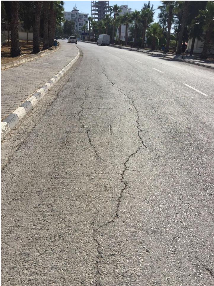
Figure 8: Example of longitudinal crack
