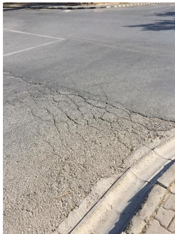
Figure 4: High severity alligator crack
