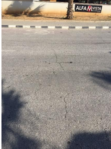
Figure 10: Low severity transverse crack
