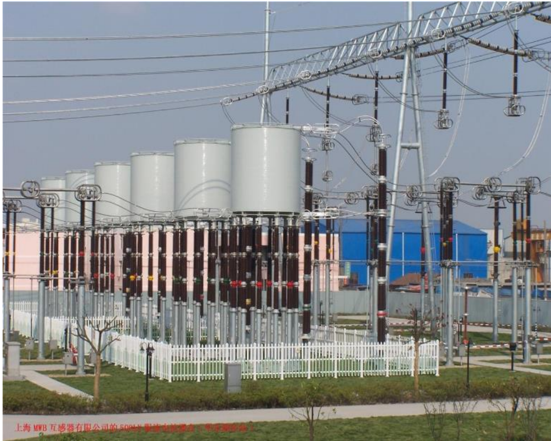
Figure 5. The Sijing 500 kV substation (Cigre Comite Chileno)
