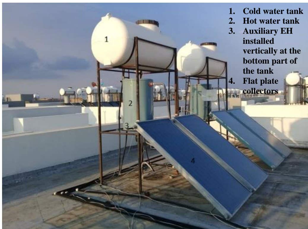
Figure 1: View of the solar/electric water heating units in Cyprus
