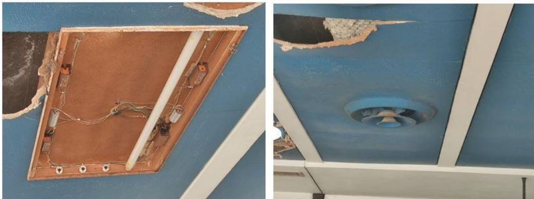
Figure 75: Ceiling Fixtures (Photo: Abraşoğlu, M. 2022).
