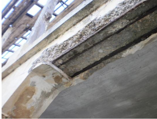
Figure V- 42: Visible concrete and steel in the construction of veranda in House 3 (Author, 2012)
