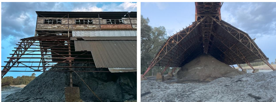
Figure 13: Material Loss on Roof & Hazard (Photo by Author, 2024)
