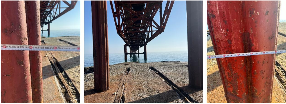
Figure 17: Rust and Corrosion on Steel Columns (Photo by Author, 2024)
