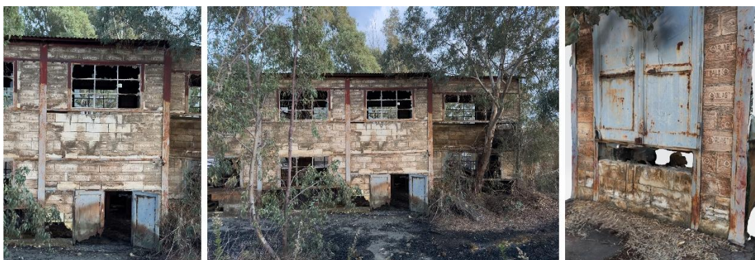
Figure 16: Wall Material Decays & Broken Windows (Photo by Author, 2024)
