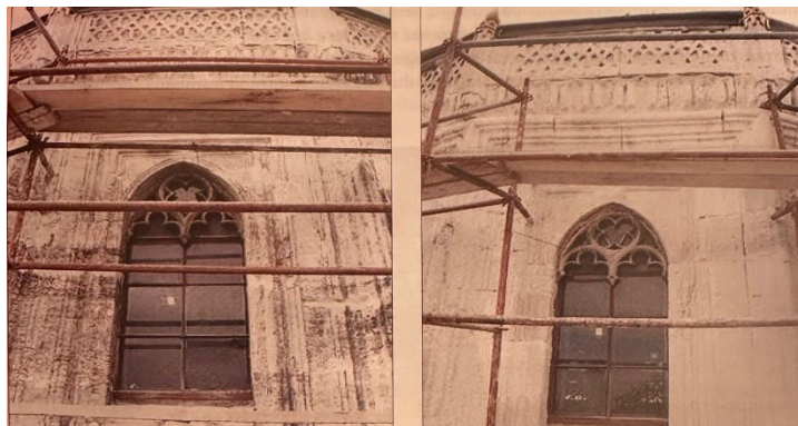
Figure 9: Pertevniyal Valide Sultan Mosque pressure washing cleaning before and after (Zakar & Eyüpgiller, 2015, p:119)
