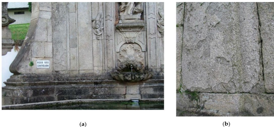
Figure 14: Example of water deterioration on the fountain of Braga (NW Portugal): (a) general view showing the position of the eroded portions to the water flow (b) detail of the erosive features (Alves et al., 2021, p:7)
