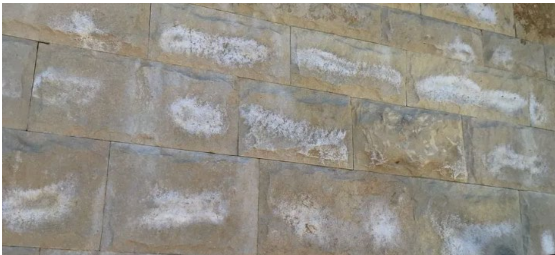
Figure 15: Efflorescence on masonry surfaces (URL 7)
