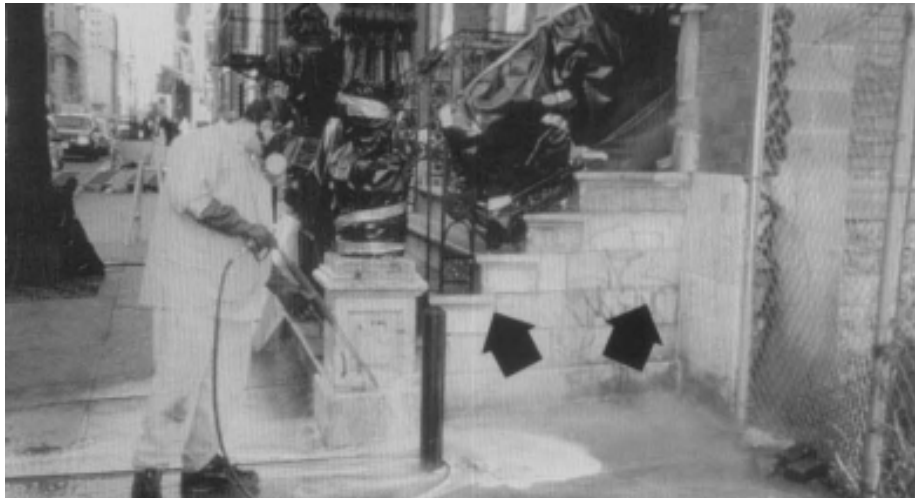
Figure 10: After cleaning with an alkaline paint remover (Weaver, M. E.,1995).
