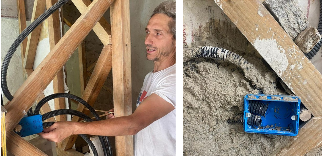
Figure 39: Placement of Electric Box, photo by author, Ghesc, Italy, 2023
