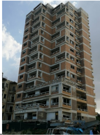
Figure 52: Shifted balcony in Twiga Tower
