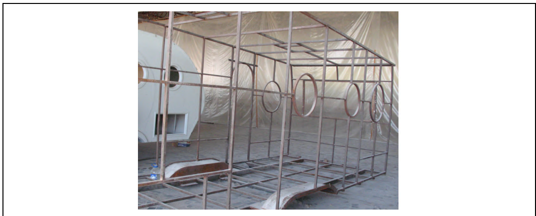
Figure 21. Steel construction prepared to be coated with composite material in abstract caravan (Source: Çelikbilek, 2019)
