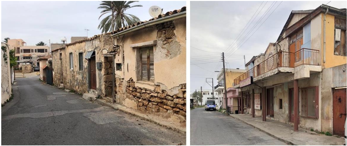
Figure 15: Physical condition of some buildings, source (Author).
