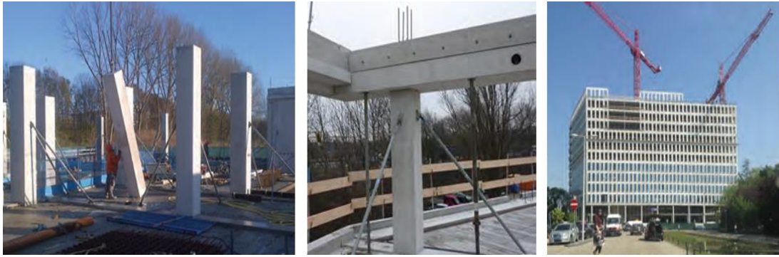
Figure 30: Efficient Construction of The Edge Comprised Prefabricated Building Assembled at Site (Jalia et al., 2019).
