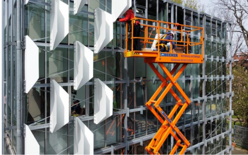
Figure 45: Initial Installation of Flectoline Modules (University of Stuttgart, Institute of Building Structures and Structural Design, 2024).
